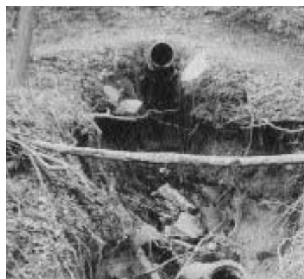
The failed storm drain on the northeast side of Wayne Road before repair work. Note the erosion and lengths of drain pipe that have fallen off as a result.
